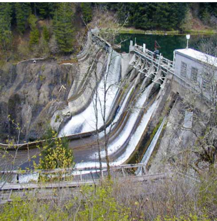
The nearly 100-year-old Condit Dam, slated for removal to allow fish passage to the upper reaches of the White Salmon River.
